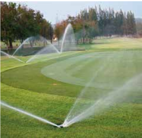
Sprinkler system on a golf course
