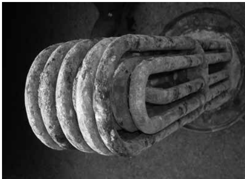
Fig 1. Heating element with scale deposits
